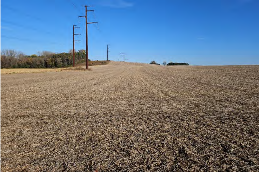
Photo 1. Overview of the North Rochester Substation expansion area from southwestern corner of expansion area facing north.
