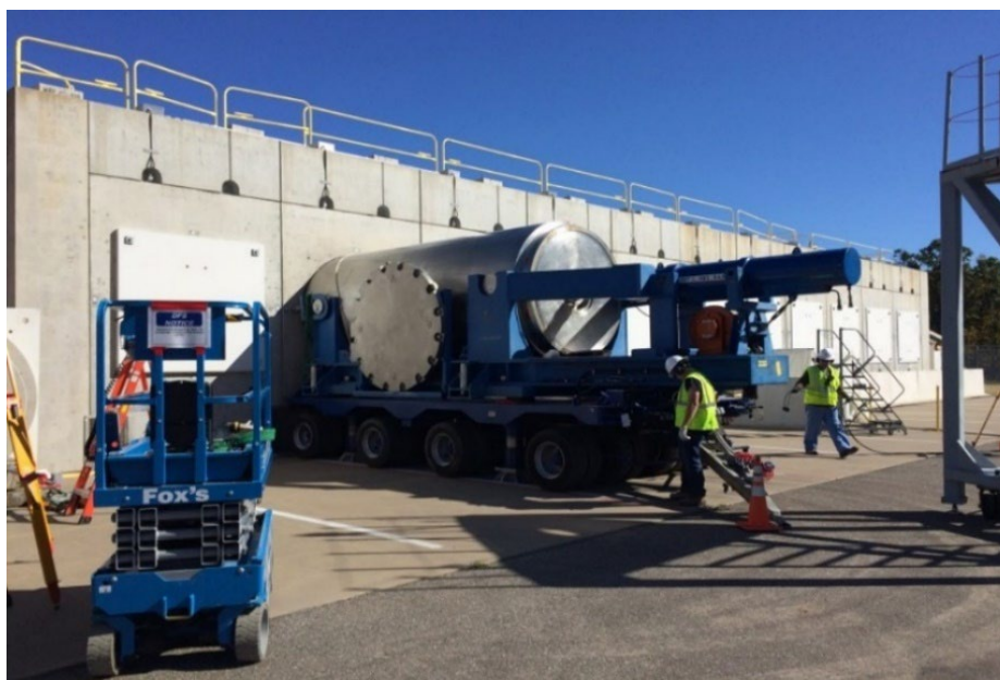
Figure 3: Placement of Canisters in Horizontal Concrete Overpack
