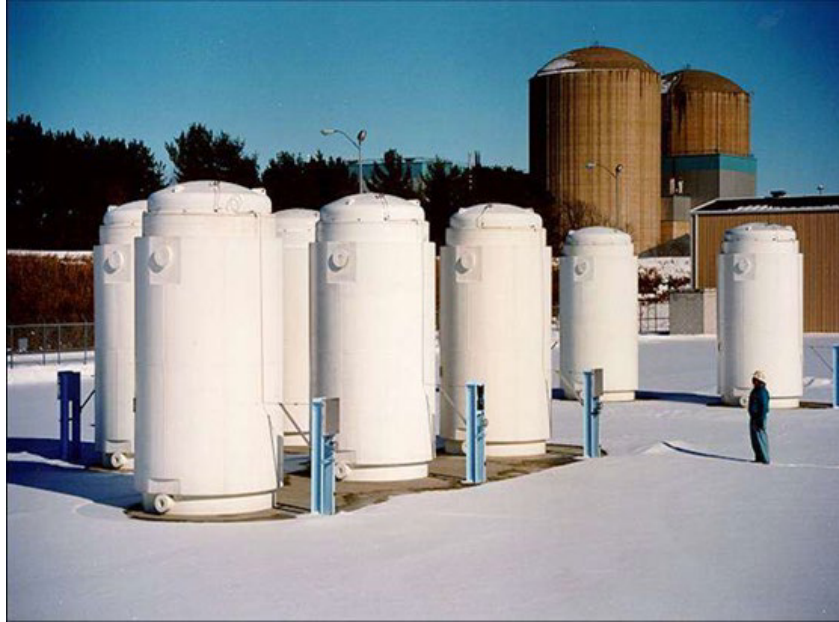
Figure 4: Current TN-40 and TN-40HT Casks on ISFSI Pad
