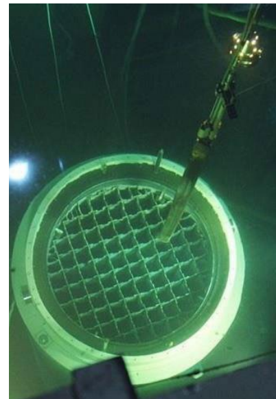
Figure 5: DFS System in Spent Fuel Pool Loading Spent Fuel Assemblies (Credit: Holtec International)
