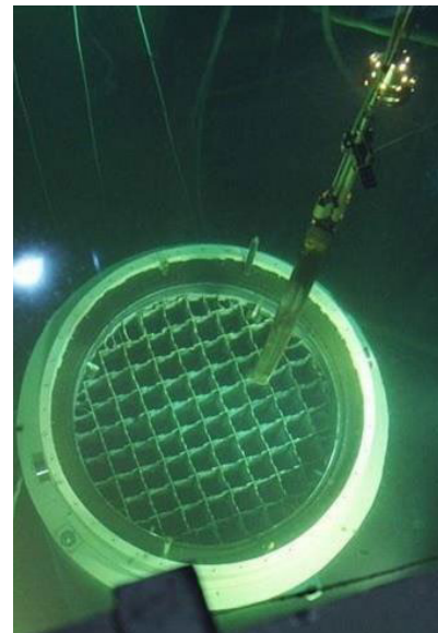
Figure 5: DFS System in Spent Fuel Pool Loading Spent Fuel Assemblies (Credit: Holtec International)
