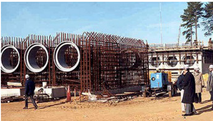
NUHOMS horizontal spent fuel storage system under construction at the Calvert Cliffs Nuclear Power Plant in Lusby, MD.
