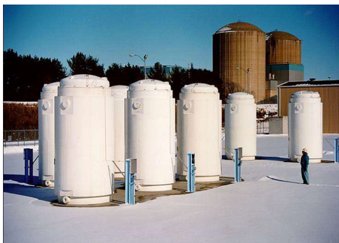
Figure 4: Current DFS on ISFSI Pad
