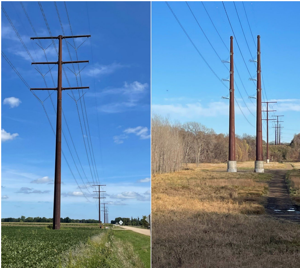
Typical Double Circuit Structures | Typical Dead-end Structures
