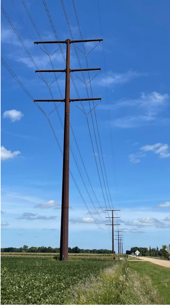
Double-circuit tangent structure
