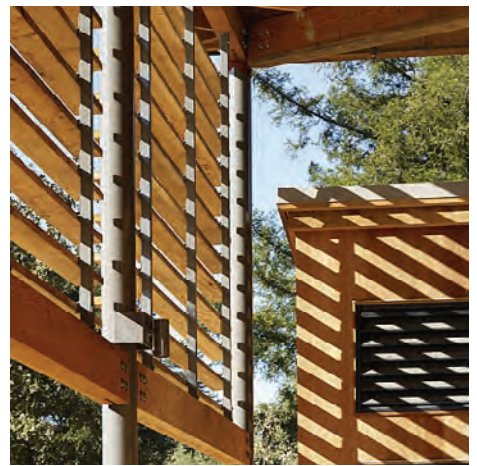
Solar control devices should not interfere with the transparency of a building facade.
