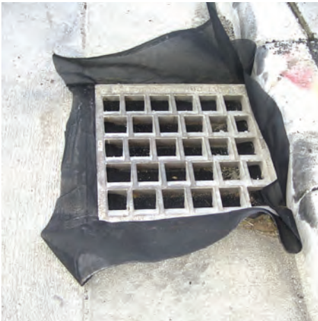
Storm drain protection
