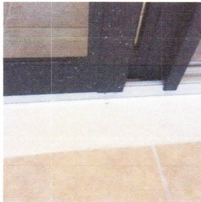
Figure A2: Newly installed sliding door at unit 209 that was not properly flashed
