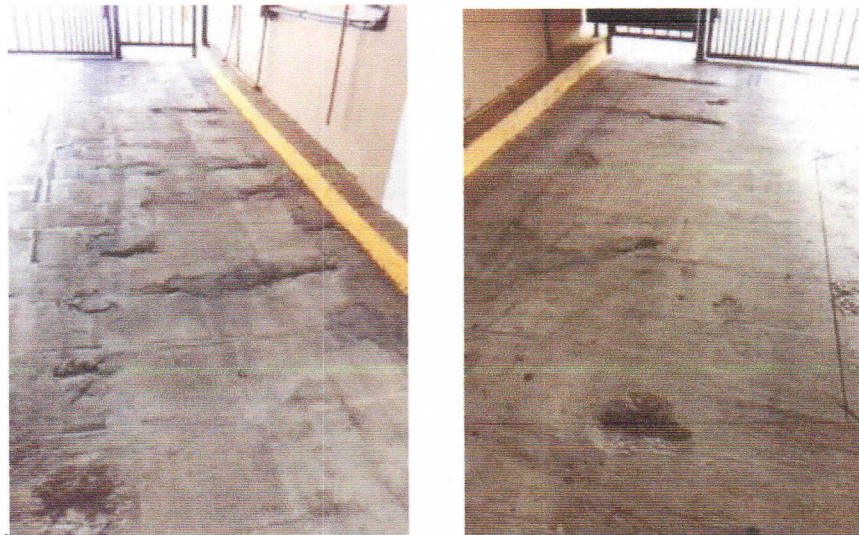
Figure J2: Spalling with exposed steel reinforcement at topside of garage deck.
