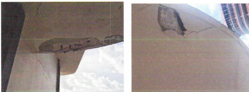
Figure C: Concrete spall at balcony slab edge in units 1008 & 211
