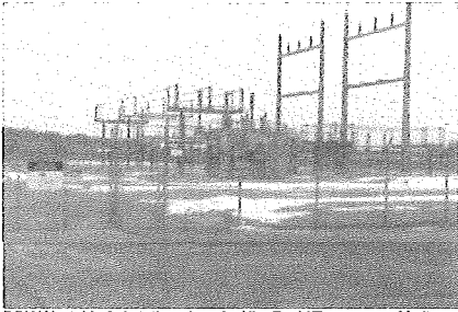
RPU Westside Substation-photo by Kim David/Townsquare Media
