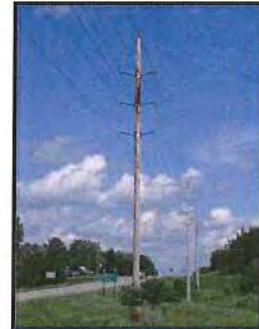
Typical 115 kV Wood Double Circuit Structure
