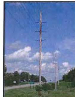
Typical 115 kV Wood Double Circuit Structure
