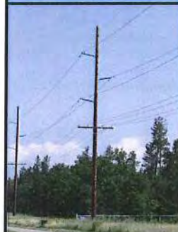
Typical 115 kV Wood Structure with Distribution Underbuild
