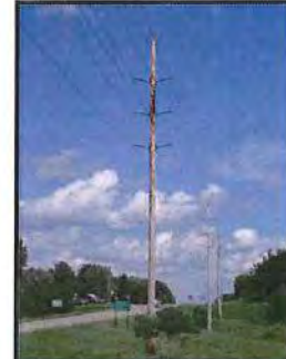
Typical 115 kV Wood Double Circuit Structure
