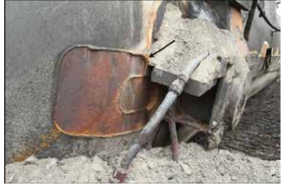
Photo 18. Damaged stub sill
